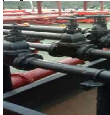
Gambar 6 Manifold bunker disegel
