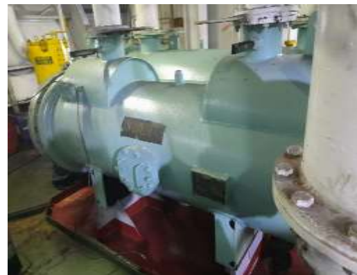
Gambar 4. 3 Fresh Water Cooler
